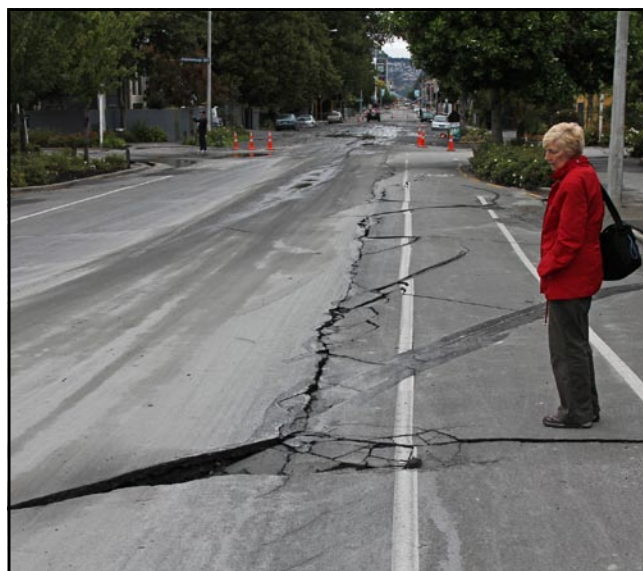
Figure 8. A cracked road in the city centre.
