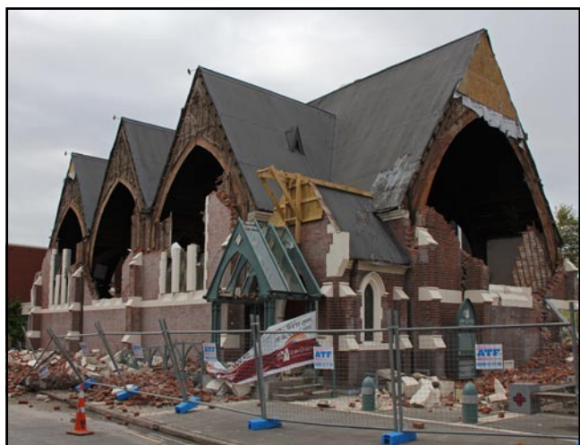
Figure 6. A church that was damaged by both the earthquakes that struck Christchurch, in February of 2011 and in the previous September.
