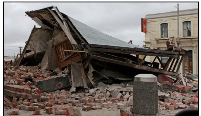
Figure 5. Total destruction of a brick building along the main road into town.
